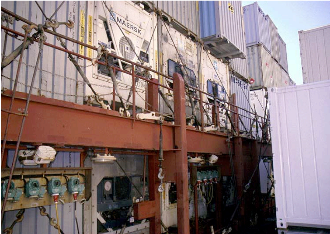
The “reefer bay” on a major container vessel. The reefer bay holds the electric supply for the individual reefers onboard.
